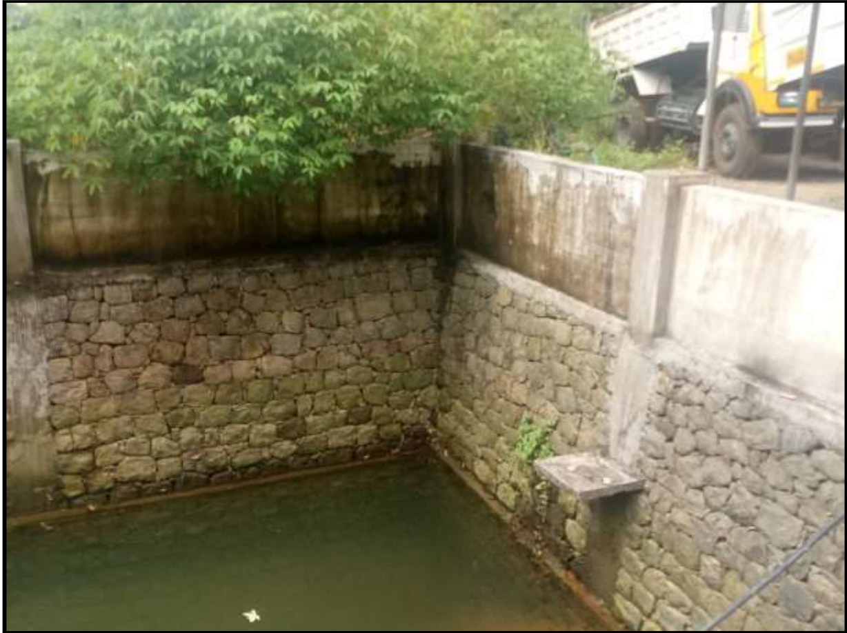
Photograph showing the rain water harvesting tank
