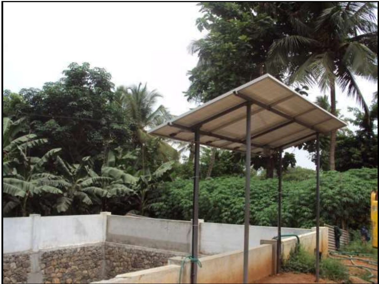
Photograph showing solar panel installed in the project area
